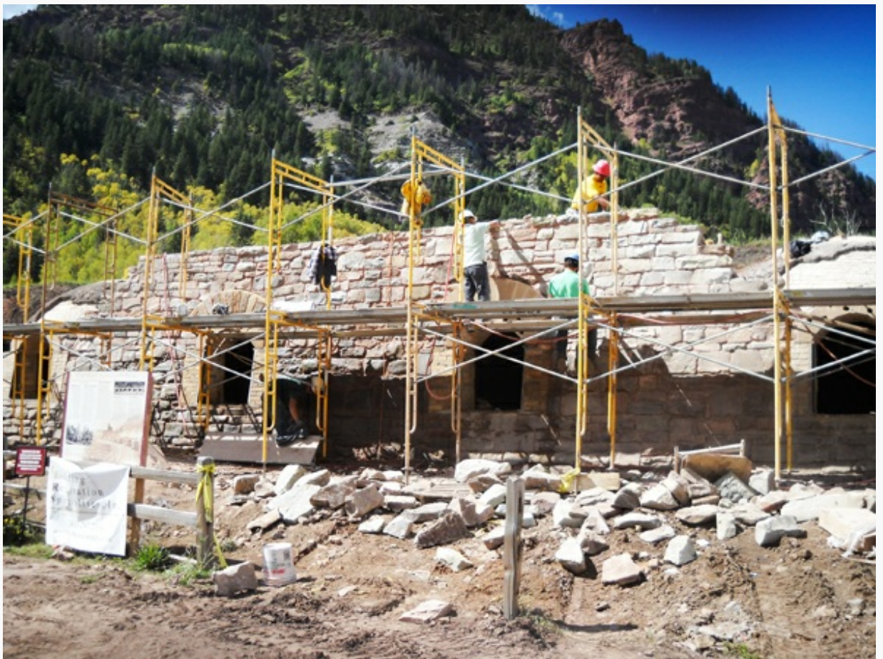
Committed to authenticity, BRS tracked down the appropriate stone and firebrick material to rebuild the ovens and the stone wall fronting them.
