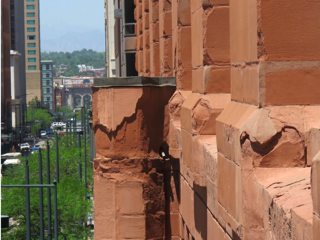
Photo courtesy of BRS. Stone and flashing showing wear on the Brown Palace Hotel.
